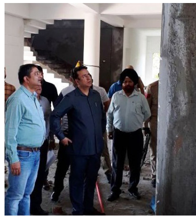
completed soon and work of slab of 2nd floor, Block 'B' is in full swing and would be completed at the end of this month. Zulfkar directed the executing agency to accelerate the pace of work so that the prestigious project is completed well in time. He said that with its completion,
